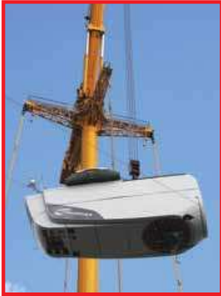
Nacelle housing gearbox and generator being hoisted during installations (courtesy of Nordex)
